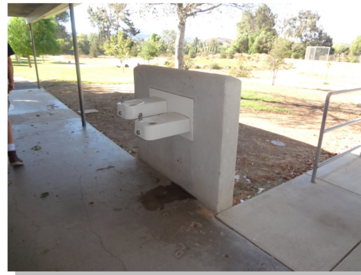
Photo -3 The drinking fountains are not current with accessibility standards.
