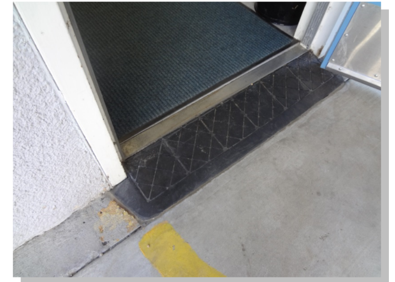
Photo -2 Typical door thresholds are not current with accessibility standards.
