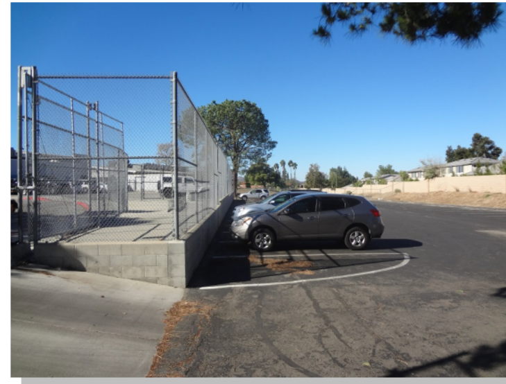
Photo -1 The site has an additional parking lot that was converted from the old basketball court. This parking lot has not been made accessible
