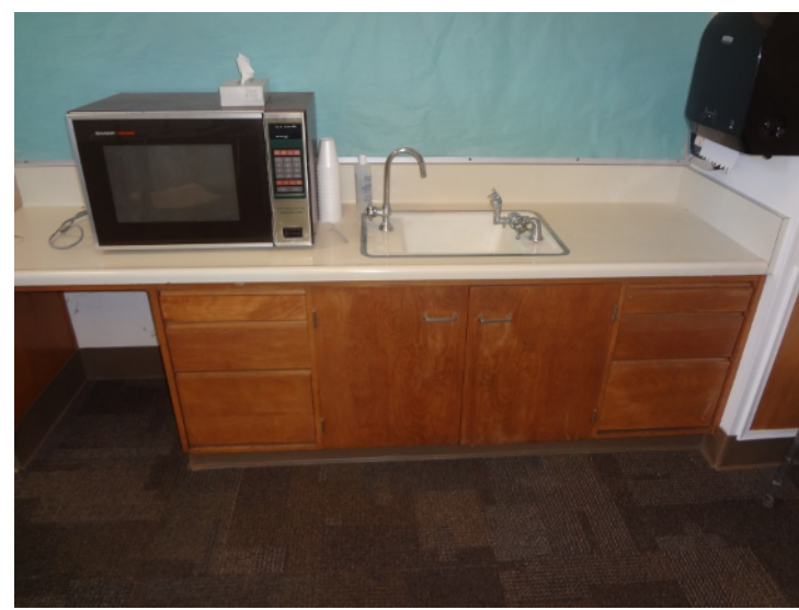
Photo -10 Building 3 Typical sink in permanent classroom building. Not current with accessibility standards.
