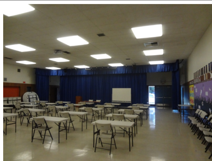
Photo -17 Building 2 Multi- purpose building is large and spacious, the flooring has some issues but is sufficient to the needs of the campus.
