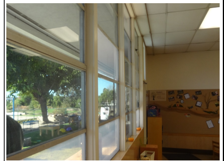
Photo -12 Building 4 Windows in typical permanent buildings are single pane and have been replaced over the years with mismatched colors of glass
