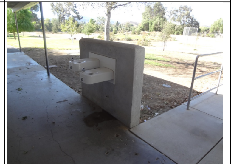
Photo -16 Building 4 Drinking fountains will need some accessibility upgrades.
