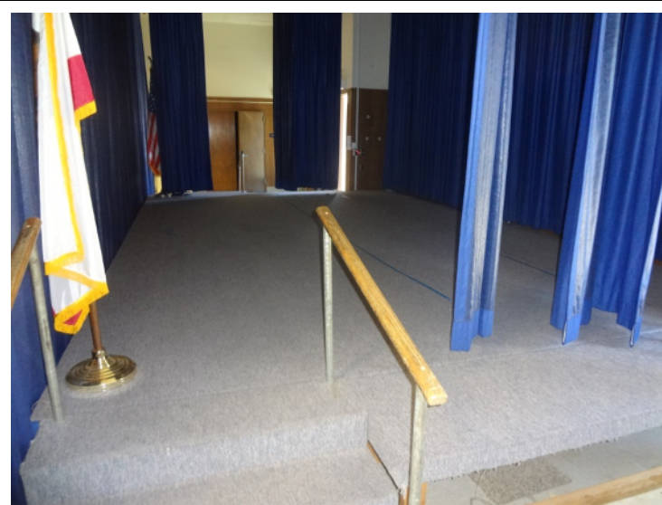
Photo -18 Building 2 Currently there is no permanent stage in the multi purpose building. A new stage should be installed.
